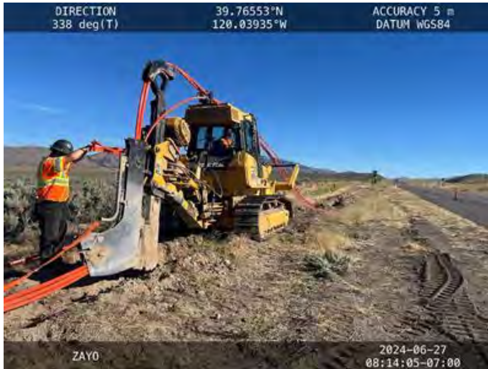
Figure 4. View to the north of plow ready to start installing conduit into pre ripped trench (Lassen County).
