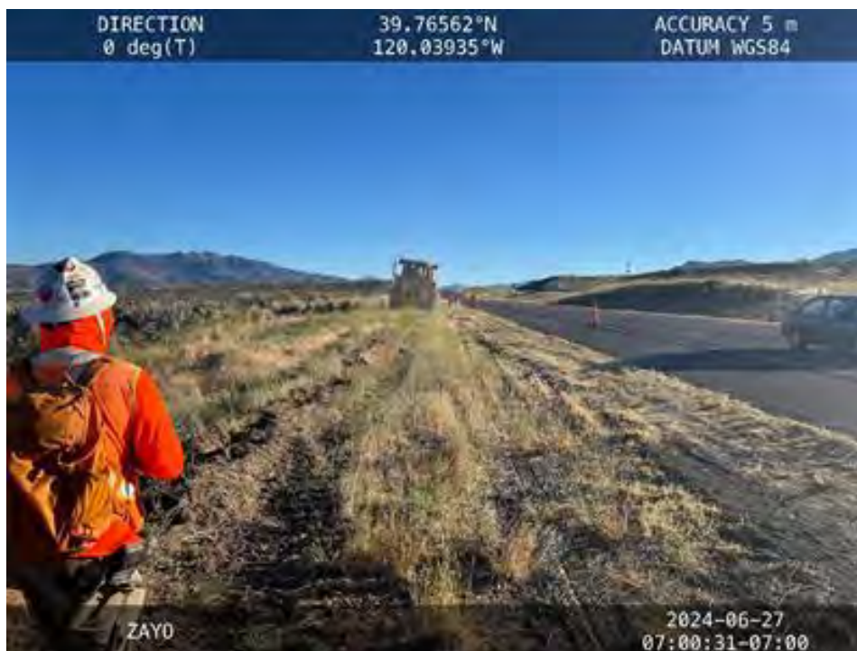
Figure 3. View to the north of pre-ripping operations for conduit install, with paleontologist monitor monitoring earth disturbance (Lassen County).
