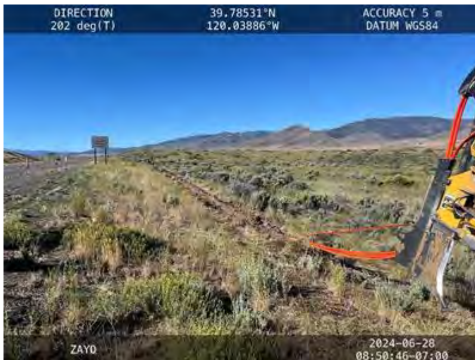
Figure 5. View to the south of conduit being plowed into the ground (Lassen County).
