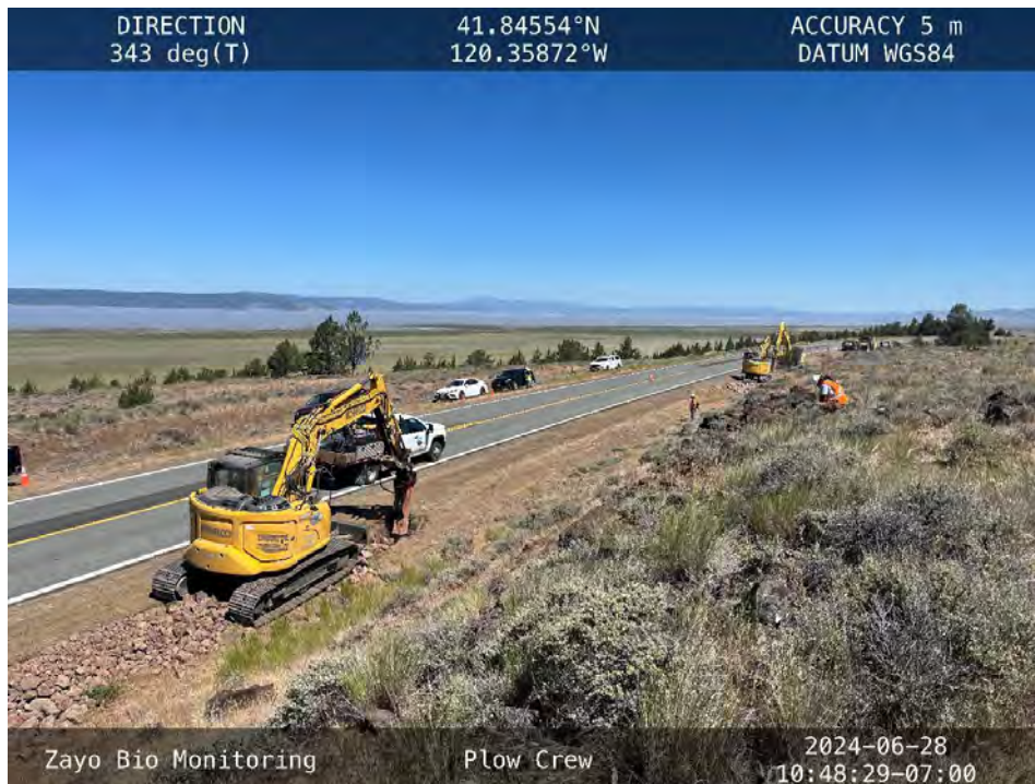
Figure 1. View to northwest of rock hammer working along fiber trench (Modoc County).
