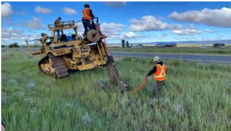
Figure 13. Overview monitoring tie-in facing southwest.
