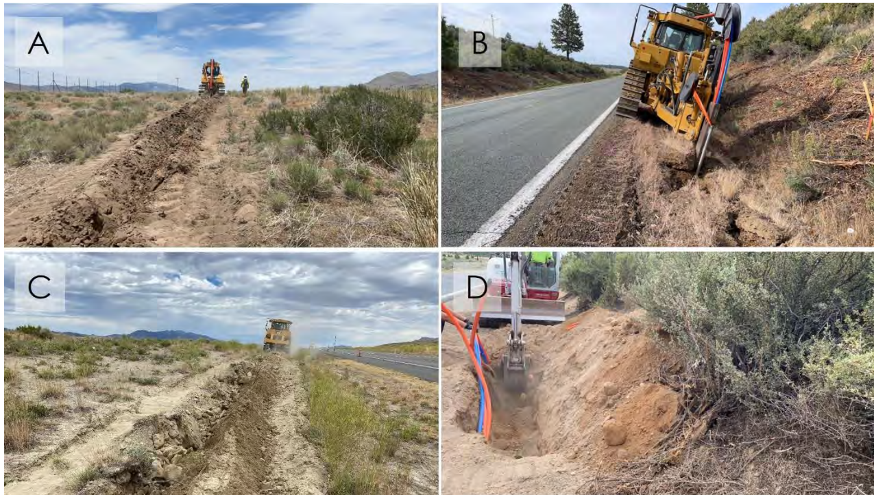
Figure 19. Overview of ground disturbing activities (selected examples): (A) overview of plowing at L-MP0.9 to 1.1, view to the north; (B) overview of plowing at L-MP2.4 to 3.4, view to the south; (C) overview of pre-plow ripping at M-MP53.8; (D) overview of tie-in trenching, view to the south.
